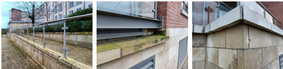
Snagging and weathering issues along Foss View (all Duncan Marks, 2024).
